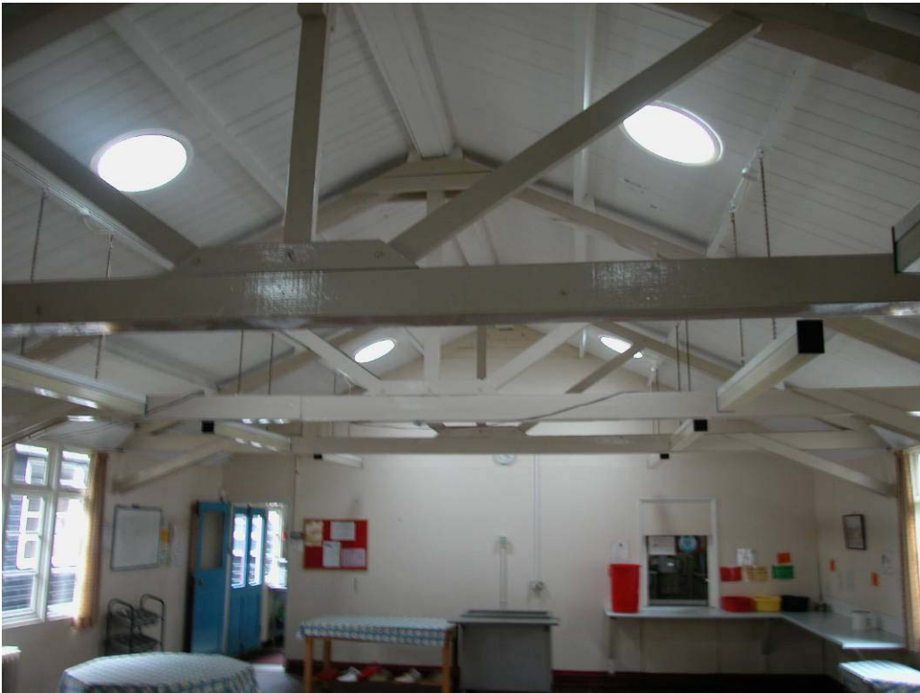
The Effect of the Sun-Pipes Inside the Building.
