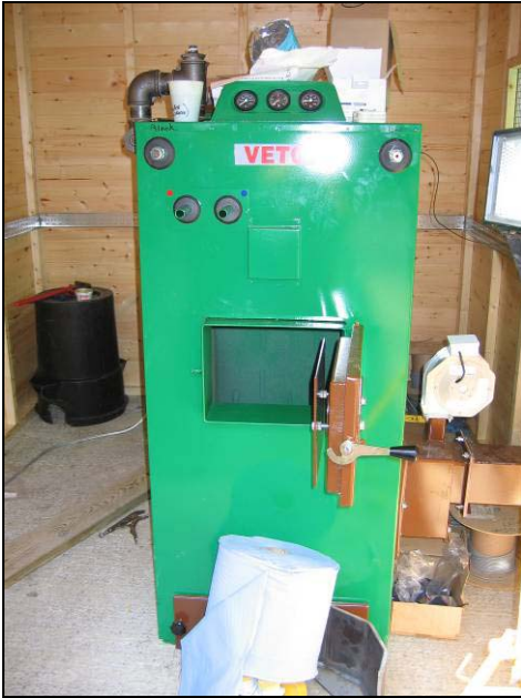
The Woodchip Boiler
