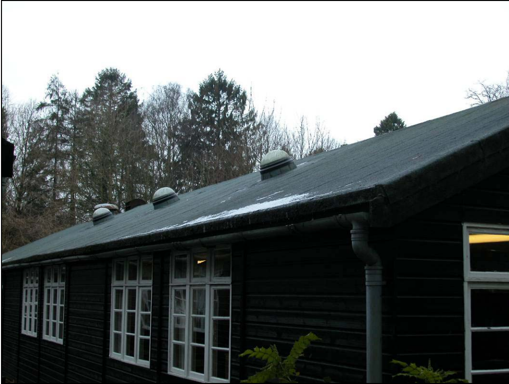
The Sun-Pipes from the Outside of the Building.
