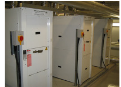
Ground Source Heat Pumps
