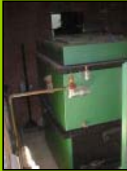
Figure 1b: Boiler and Silo
