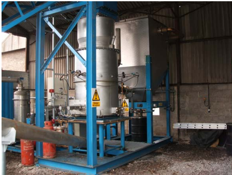
Gasifier with gas filter behind
