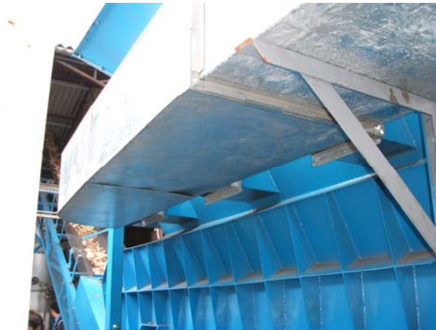
Heat from engine exhaust feeding woodchip hopper
