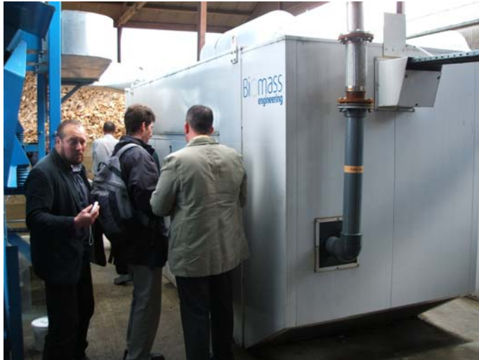
Acoustic enclosure, engine within. Gas feed shown.
