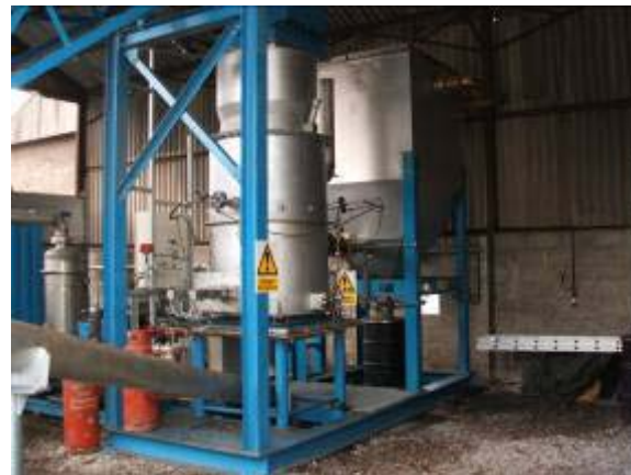
From chips to heat and electricity by gasification
