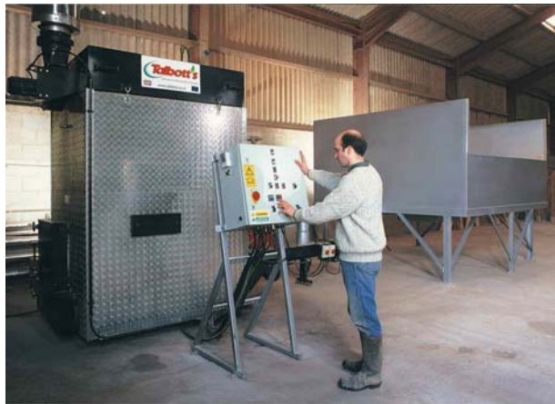
ARBRE Farmer, Gareth Gaunt, with his new Biomass Heating System
